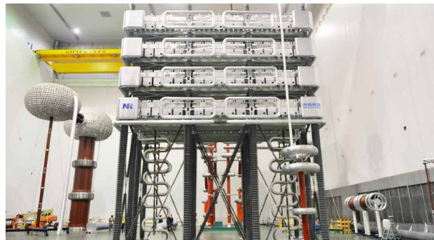
VSC Converter Valve
