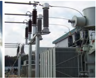
Figure. PCS-9250 AIS OCT in 110kV Dalv digital substation in Zhejiang Province
