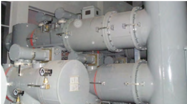
Figure. PCS-9250 GIS ECT/EVT in a 110kV digital substation in Jiangxi Province
