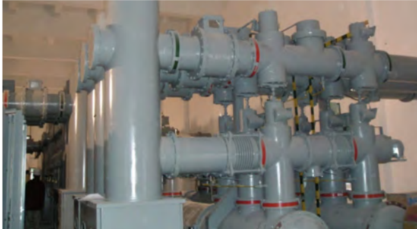
Figure. PCS-9250 GIS ECT/EVT in a 220kV digital substation in Shandong Province
