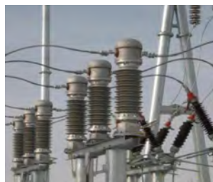
Figure. PCS-9250 AIS ECT/EVT in a 110kV digital substation in Liaoning Province
