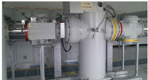
Figure. PCS-9250 GIS OCT in 110kV Huangtun digital substation in Shandong Province
