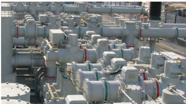
Figure. PCS-9250 GIS ECT/EVT in a 220kV digital substation in Anhui Province
