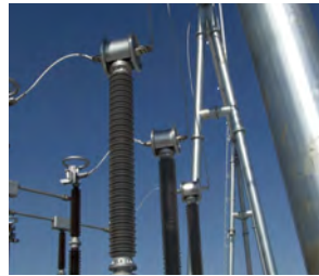
Figure. PCS-9250 AIS OCT in 220kV Jinshan digital substation in Heilongjiang Province
