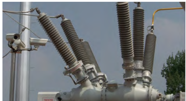
Figure. PCS-9250 GIS OCT in 110kV Zibo digital substation in Shandong Province
