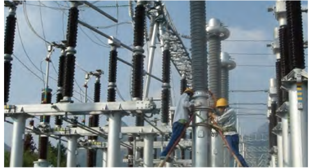
Figure. PCS-9250 AIS OCT in 220kV Lanxi digital substation in Zhejiang Province
