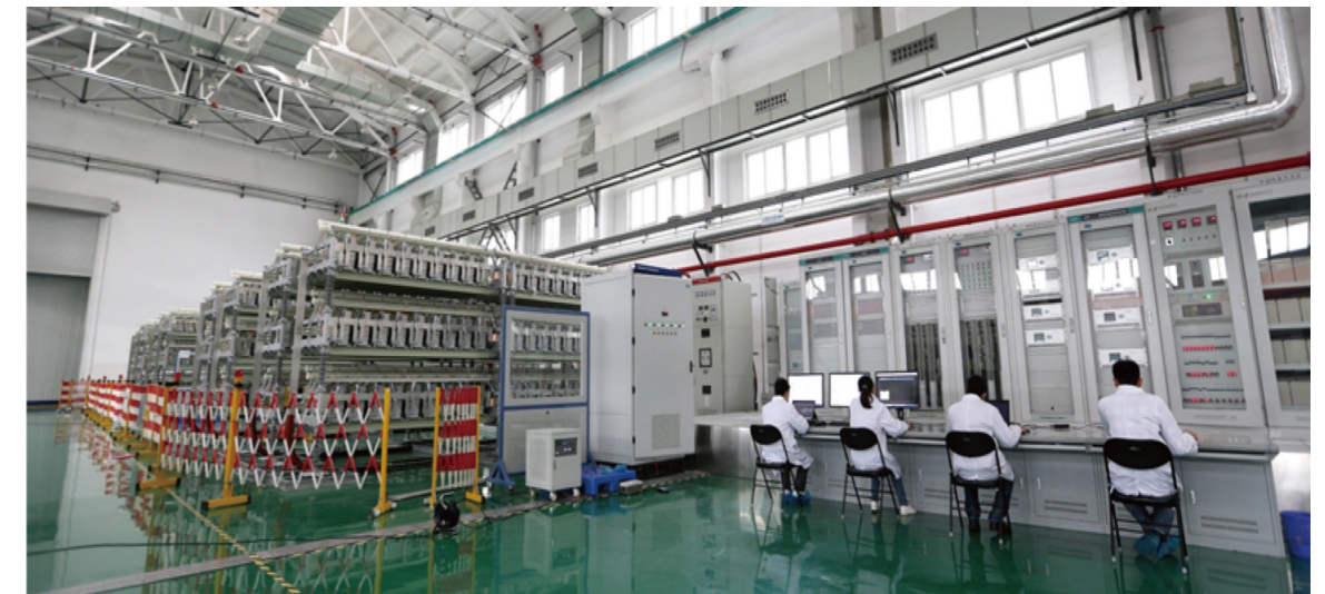
VSC-HVDC BTB test platform
