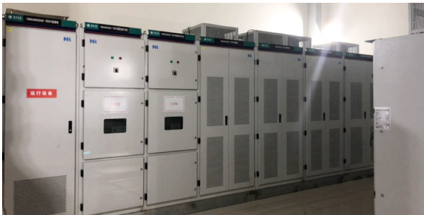
Static frequency converter picture taken on site
