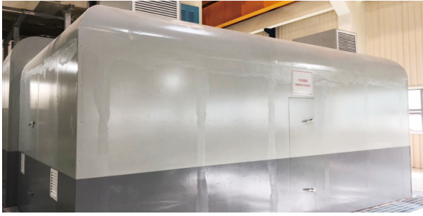
Synchronous condenser picture taken on site
