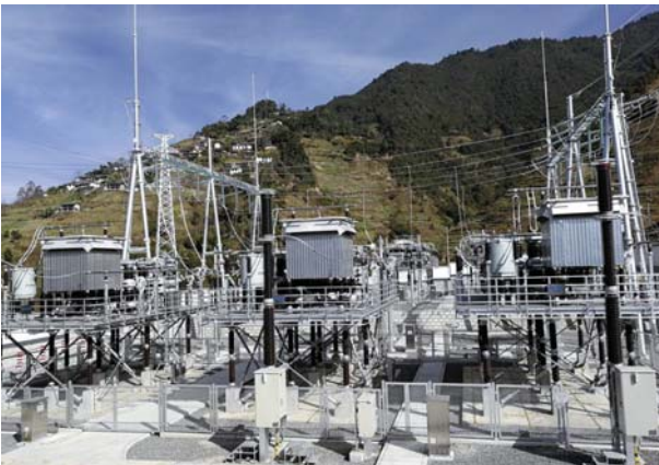
Figure 2 220kV Fixed Series Compensation Site
