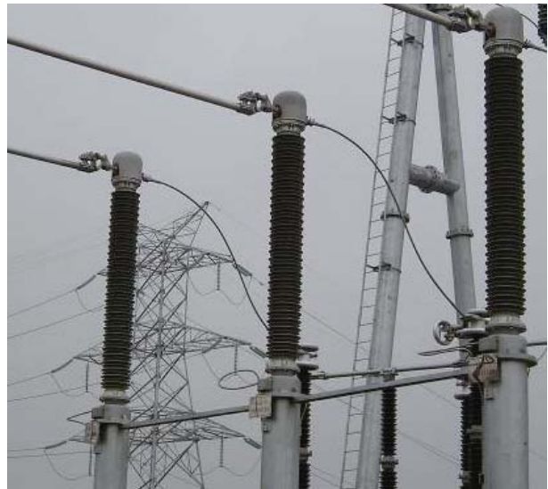
Figure 3 Electronic CT in AIS Application
