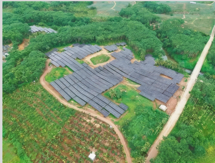
Power Generation Project Booster Station in Yangjiang Town, Qionghai 100 MW Agricultural-Photovoltaic Complementary Power Generation Project PV Array in Yangjiang Town, Qionghai
