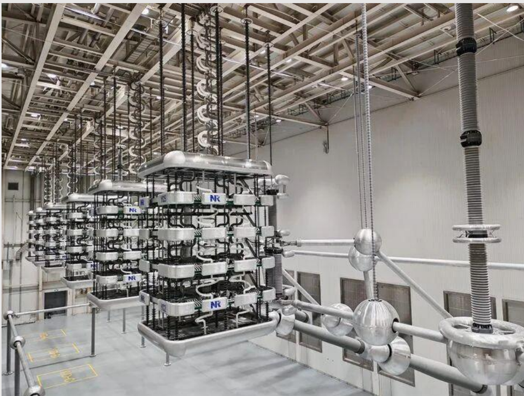
Case: NR' autonomous and controllable DCS successfully commissioned at Dadi Yuntian Chemical
