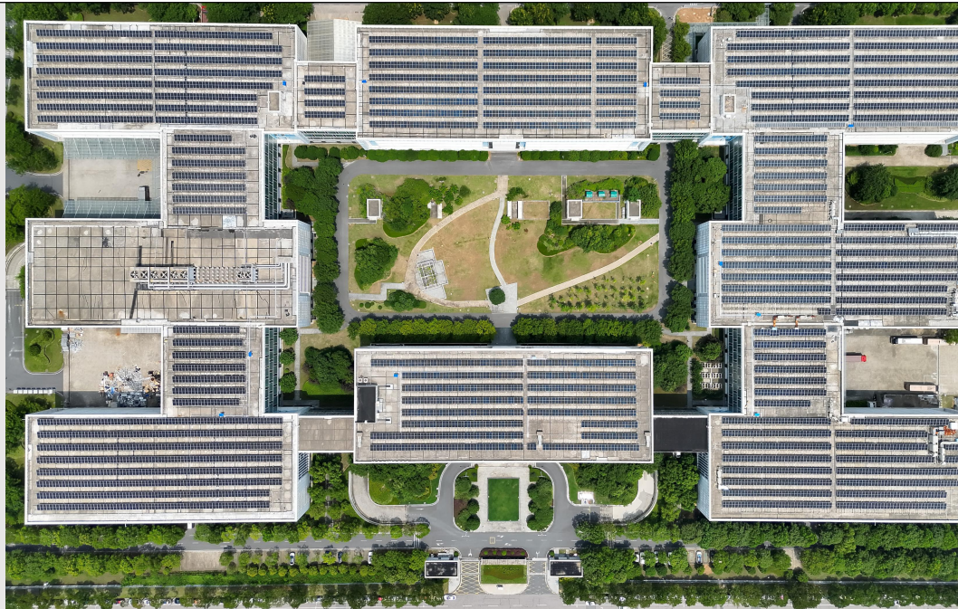
Aerial View of the Jiangjun Road Phase I Photovoltaic Power Station After Technical Renovation
