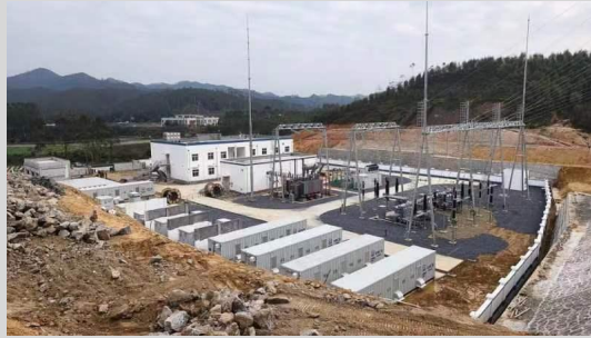
佛冈县中核汇能乡村振兴（二期）150MW 农光互补光伏项目升压站全貌 Overall View of the Voltage Boosting Station of the CNNCHN Rural Revitalization Project Phase II 150MW Agricultural Photovoltaic Project in Fogang County.
